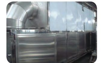
冷冻压缩机组 Refrigeration device
